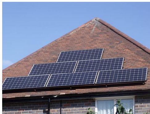
These solar panels convert sunlight into electricity.
