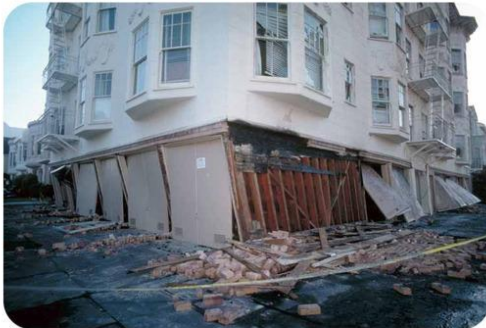
The first floor of this San Francisco building is collapsing after the 1989 Loma Prieta earthquake.
